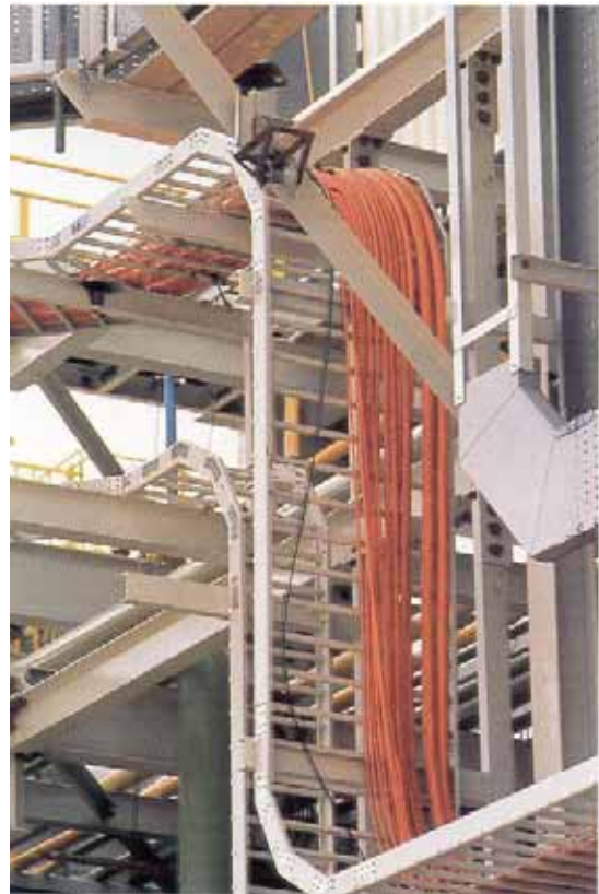
Cable ladder installation at S.C.M. Chemicals Limited's titanium dioxide Plant in Western Australia
